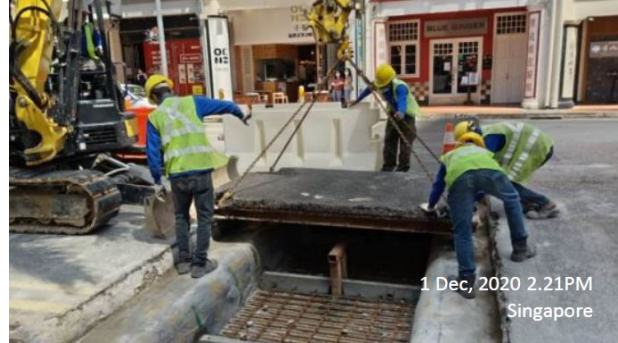
Figure 18: Laying the steel plates with 50mm thick premix and covering the trenches to allow traffic to operate.
