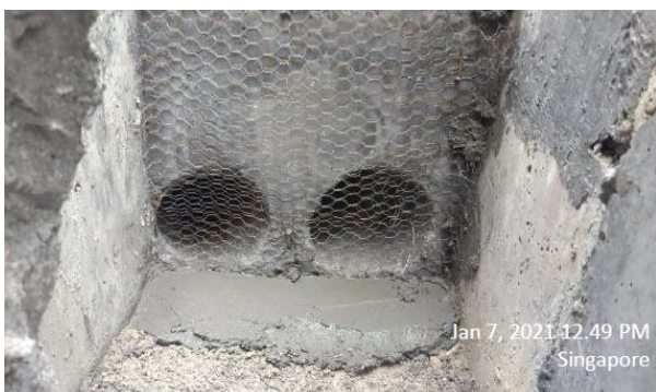
Figure 23: Casting of the concrete wall connecting the steel pipes to the drain
