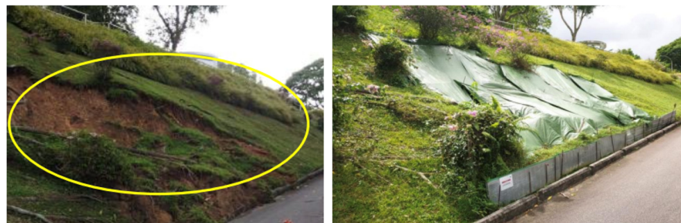
Figure 4. Failed slope (left) and mitigation work undertaken (right) in Singapore.
